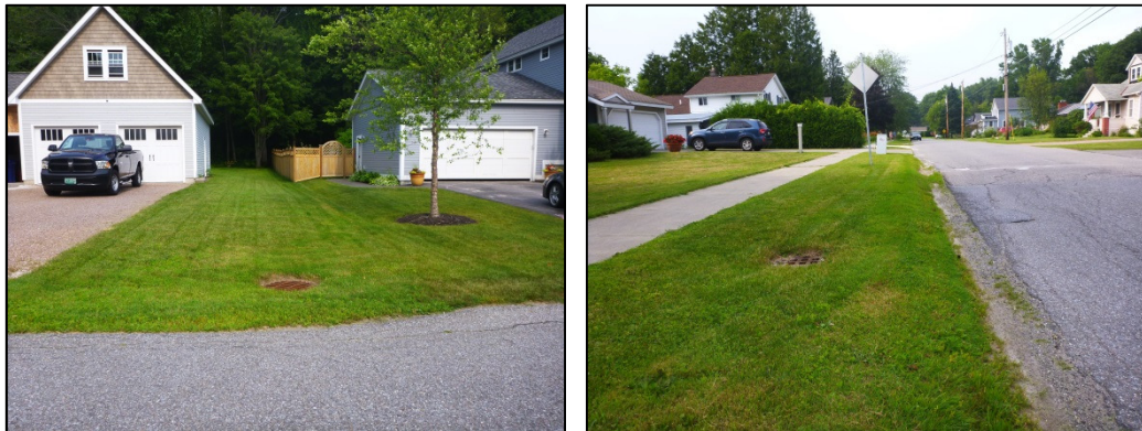
FIGURE 28. Yard drains installed within the study area, mapped as flowing into the detention pond. Note the lack of curbing. (Photos taken in July 2015.)
