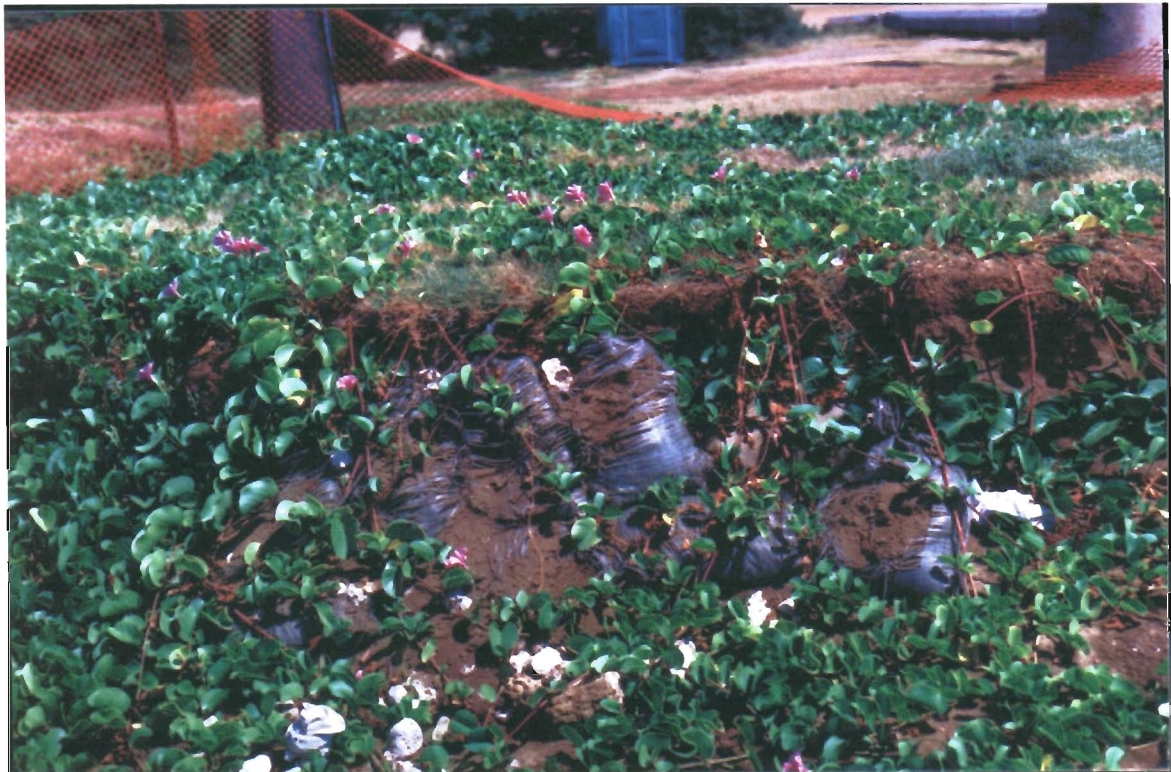
Photo 5. Fort Hase Beach Recreational Subarea. Dune erosional escarpment near picnic pavilion showing proliferation of beach morning glory Ipomoea pes-caprae .
