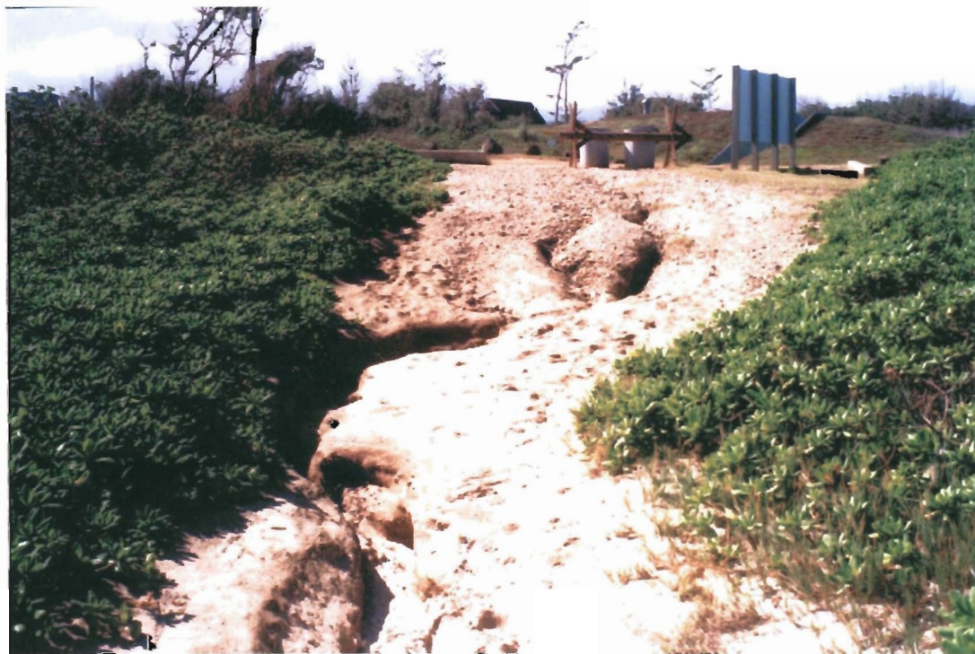
Photo 17. Pyramid Rock Recreation Subarea. Note severe erosion along beach access path from parking lot. Path is subject to runoff from the parking lot during heavy rains as well as chronic flows from the shower.
