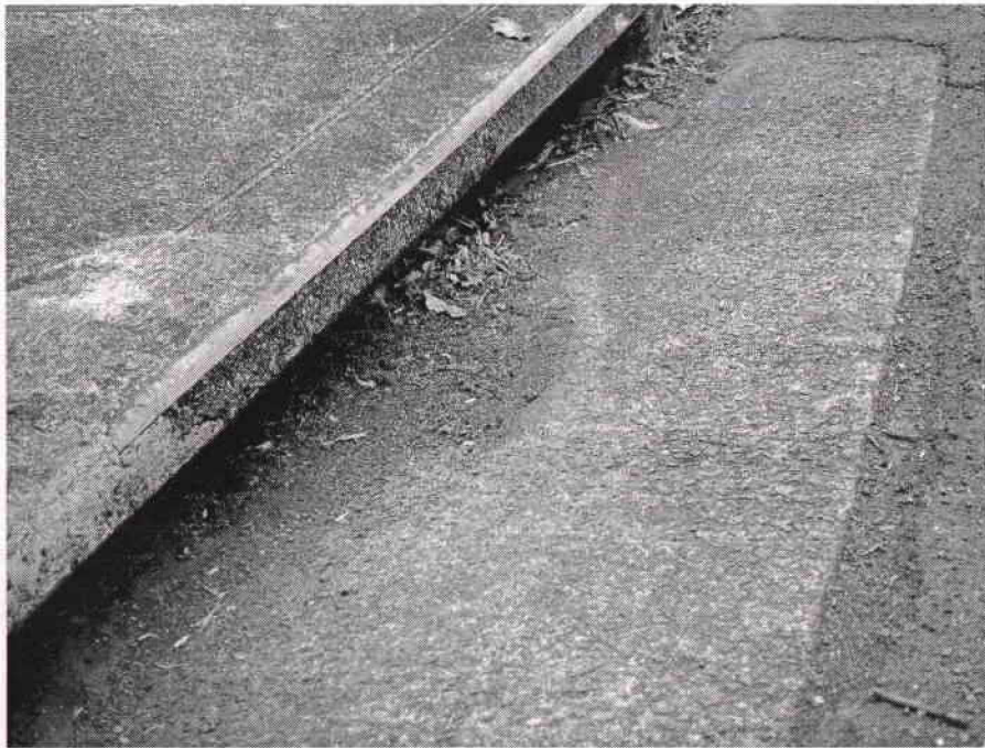
Appendix O. Road deposited sediment (RDS) near 10 th Ave. Bridge near Palolo Pl. Location south side of 10 th Ave. looking downstream
