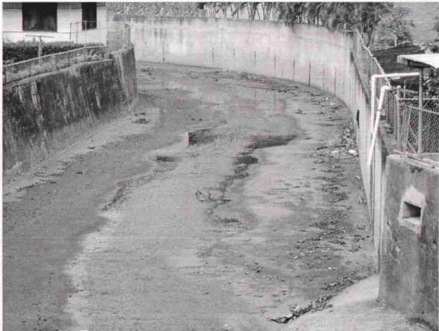
Appendix I. Palolo Stream channelization showing some sediment lag deposits along channel sides. View looking downstream from Palolo Ave. Bridge near Kehau Pl.
