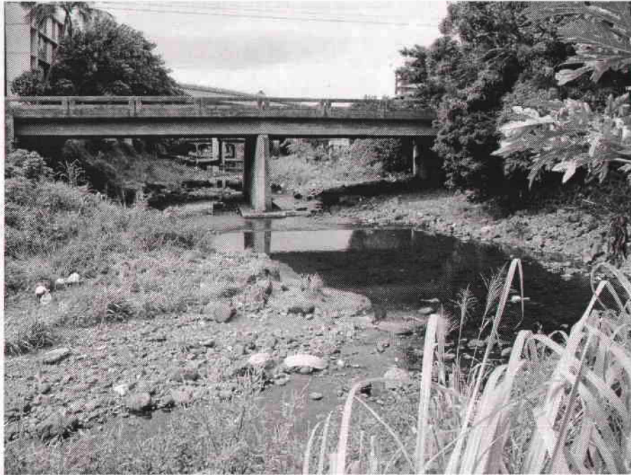
Appendix B. Manoa/Palolo Drainage Canal showing several bridges crossing the canal. View from Palolo Stream bank looking downstream
