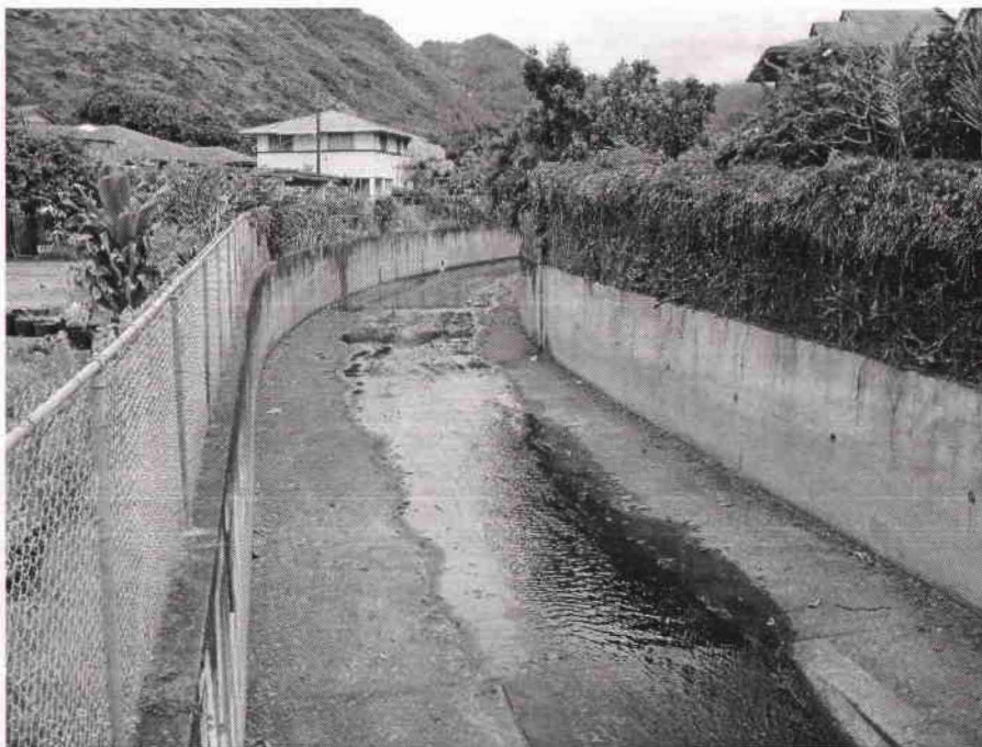
Appendix K. Palolo Stream box channelization showing storm drains along right side. View looking upstream from Paalea St. Bridge
