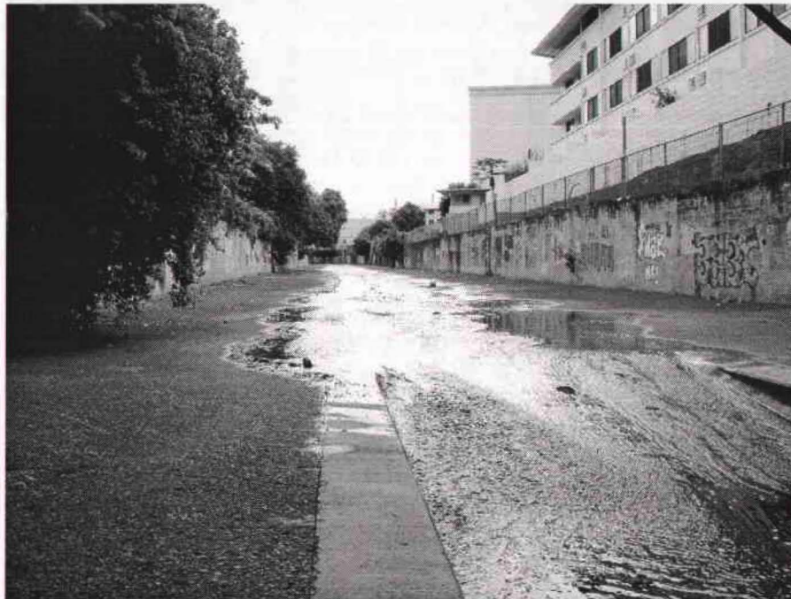
Appendix F. Palolo Stream box channelization at drop structure. View below Koali Rd. Bridge looking upstream
