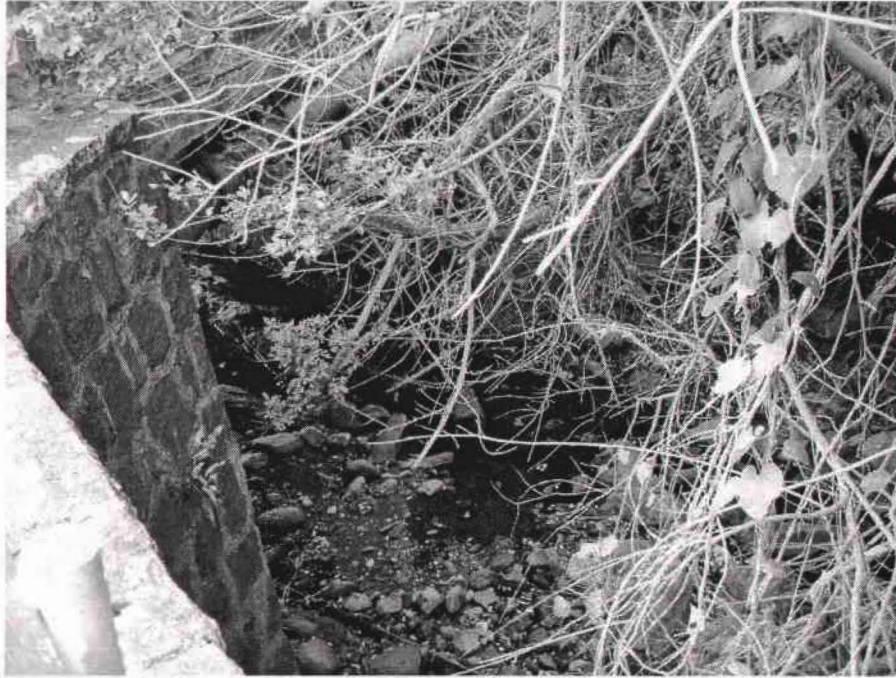
Appendix R. Waiomao Stream semi-natural channel. View from under 10 th Ave. Pl. Bridge looking upstream
