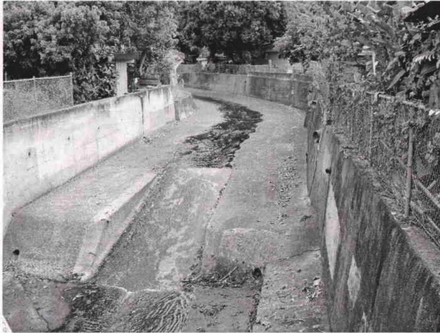
Appendix J. Palolo Stream channelization showing storm drain outlets and drop structure. View looking upstream from Palolo Ave. Bridge near Kehau Pl.
