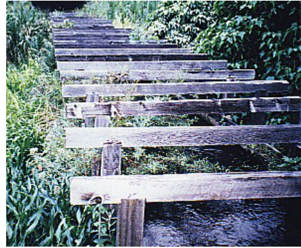
The Lower Hāmākua Ditch: wooden flume section overgrown with vegetation (October 1998).
