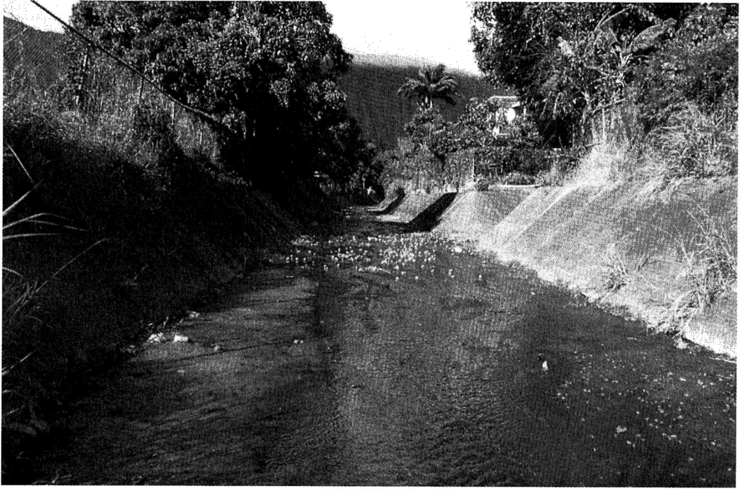
FIGURE 2. Hardened portion of Kahawai Stream just above station 16 (Figure 1).
