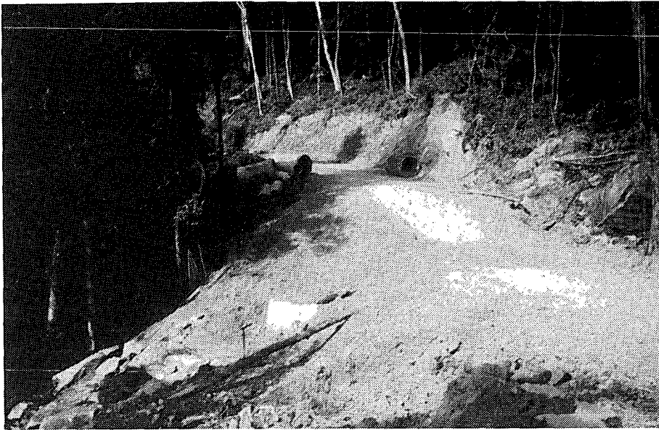
FIGURE 18. Gullying and landslips are frequent after heavy rain especially on steeper road sections. Potential remains for complete slope failure and massive sediment yield.
