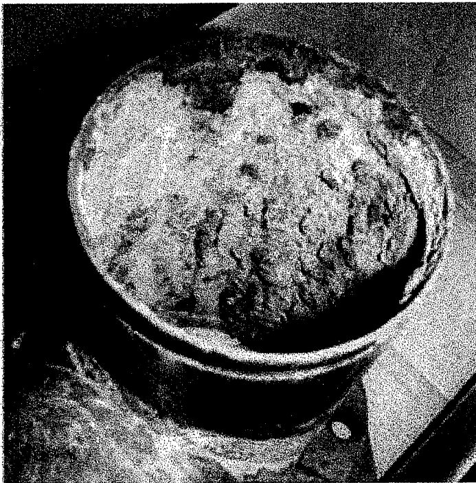
Figure 3 Tubercle growth in a FPS piping (The American Fire Sprinkler Association)
