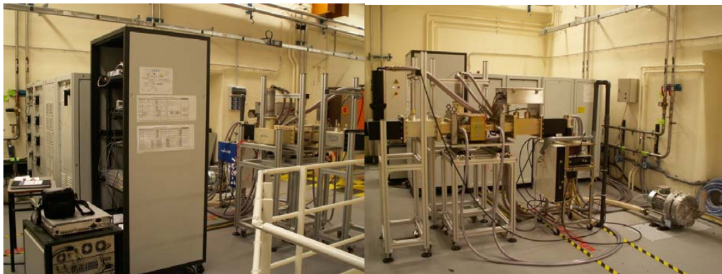
Figure 2.3: View of the RF Power supply setup at Orsay: on the left, the DC power generator as well as the 1 kW amplifier, the interlocks and control closet; on the right, a back view of the IOT with its circulators and all the pipes circuits for air and water cooling.
