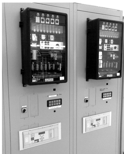
Fig. 24. Distance protection of lines based on MPD type MiCOM P437 (bottom) and on electromechanical type LZ-31 (top) connected in-parallel
