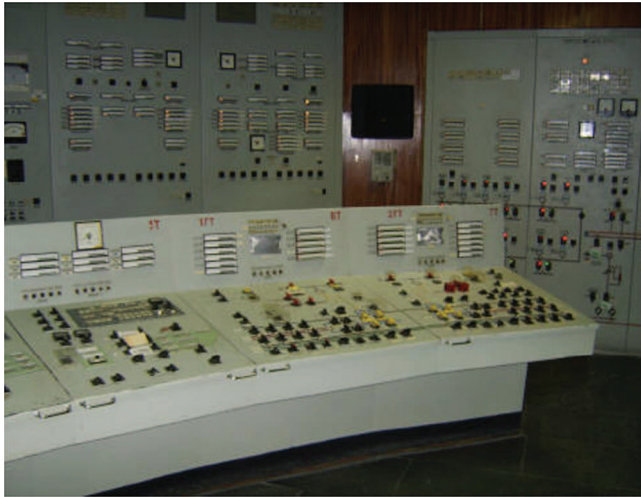
Fig. 1. Small portion of Chernobyl nuclear power plant control room (from http://www.upandatom.net/Chernobyl.htm ).
