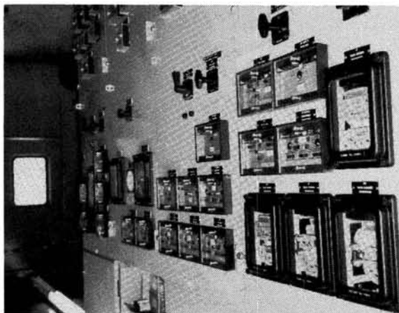
The power plant control room at the Puna Geothermal Facility.
