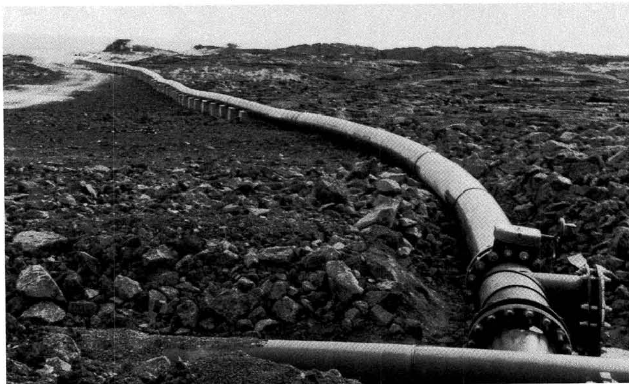
The newly installed 18-inch diameter emergency back-up pipeline snakes across the lava towards the sea. This pipeline will deliver 3000 gpm of deep cold seawater to NELH projects.
