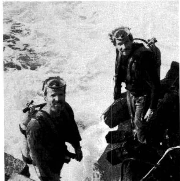
Kent Merrill (left) and Jan War (right) prepare to jump into the foamy brine to secure underwater connections at the offshore pump station.
