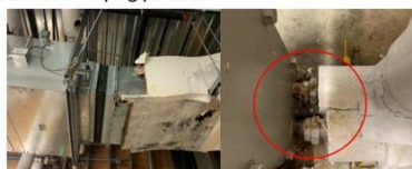
Fig. 2. Damage in mechanical penthouse
