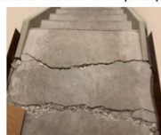
Fig. 1. Crushing of concrete at stairs
