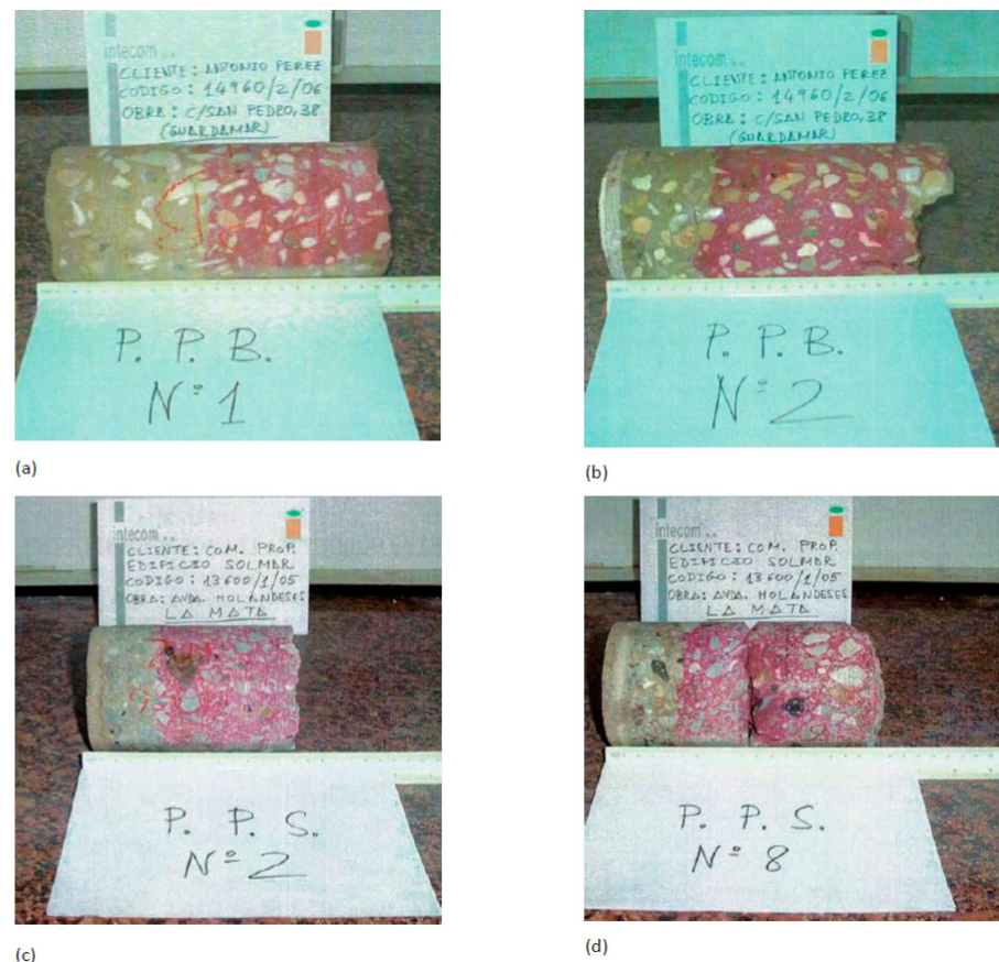
Figure 3. Depth of carbonation. (a) Building 2 Pillar 1. (b) Building 2 Pillar 2 (c) Building 4 Pillar 2. (d) Building 4 Pillar 8.
