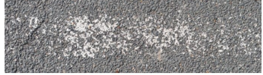
Fig. 10: Old road marking with time wear
