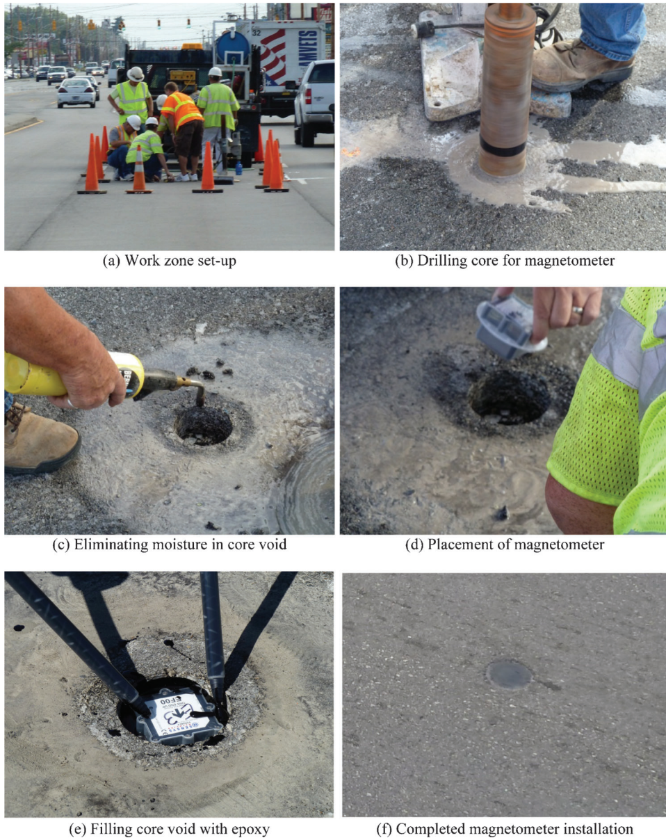
Figure 3.1 Wireless magnetometer installation. (a) Work zone set-up. (b) Drilling core for magnetometer. (c) Eliminating moisture in core void. (d) Placement of magnetometer. (e) Filling core void with epoxy. (f) Completed magnetometer installation
