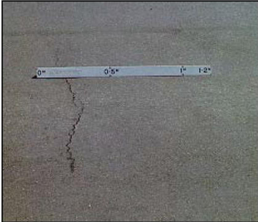
(Direction of Travel →) Figure 3: Transverse Cracking
