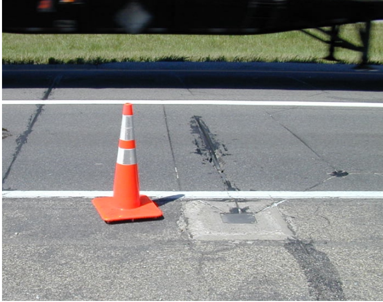
Figure 3-2: Piezo-electric WIM in pavement on I-65 NB, near Lafayette, IN
