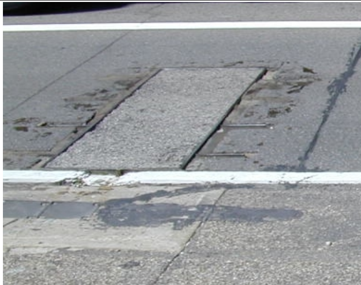
Figure 3-7: Failed Bending Plate Installation at WIM 5450 Filled with Asphalt
