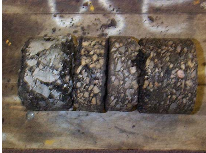
Figure E-5 Pavement Core on Southbound SR29
