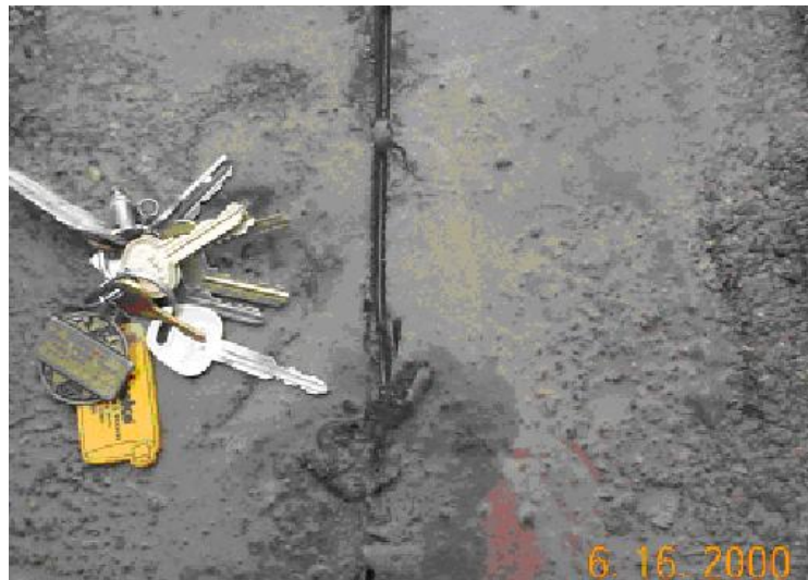
Figure 6-16 Crack after Cut
