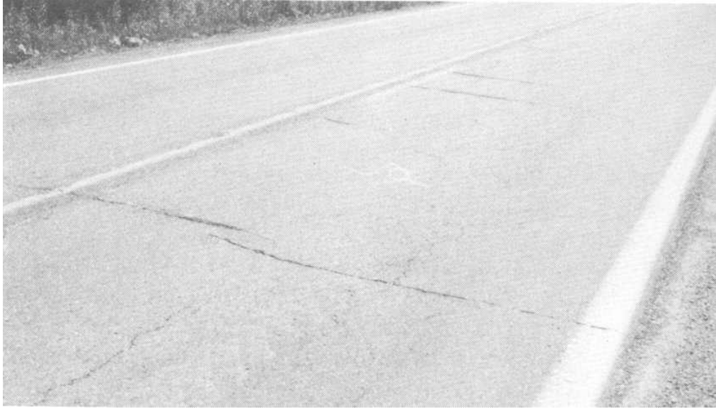
Figure 2.1 -- Thermal cracking observed in an HMA pavement (4)
