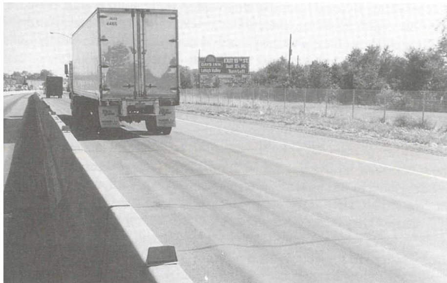
Figure 2.2 -- Rutting observed in an HMA pavement (4)
