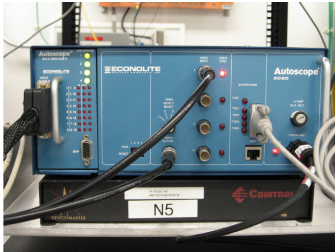
Figure 4.5 Autoscope 2020 Device in I-65 mm128 communications hut
