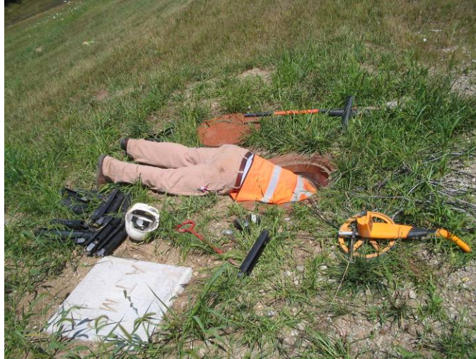
Figure 8.3 3M Microloop Sensors Placed Too Deep Below Pavement
