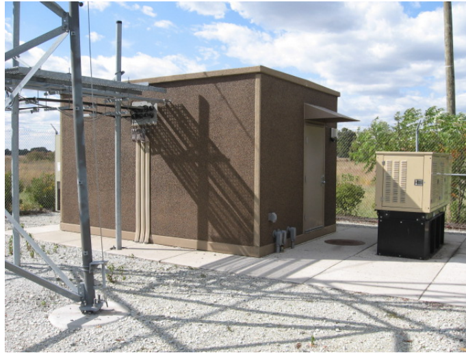
Figure 4.3 ATMS Communications Shed @ mm 128 on I-65
