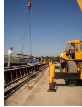
b) Setting of web and top flange portion of the reinforcing cage
