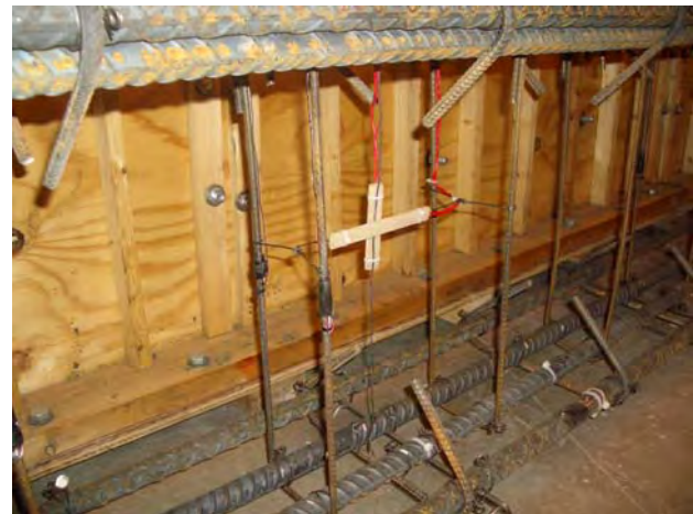
Figure 3.23 Detail of embedded concrete gages
