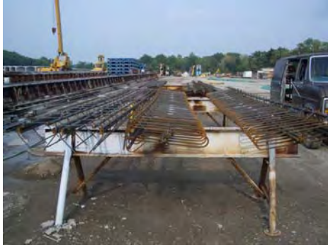
a) Bottom flange portion, and web and top flange portion of the reinforcing cages
