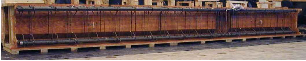
a) View of reinforcement of beam for Specimen 13.3-2.6-98 and Specimen 13.3-5.4-98 before cast
