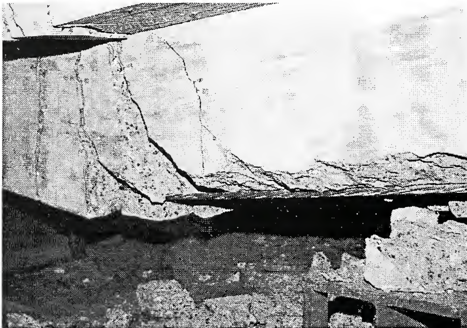
Figure 3.5-6 Exposed strand associated with bond failure in T-Beam FWC.
