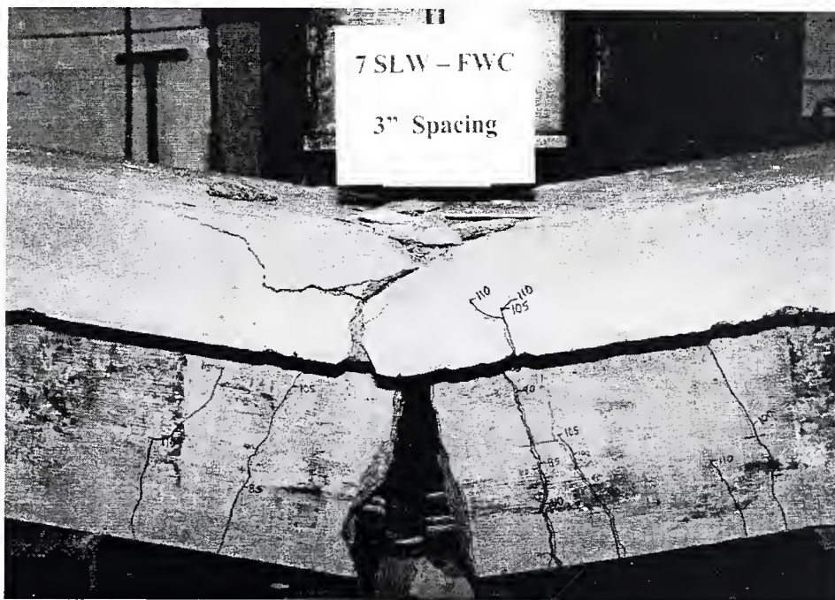
T-Beam FWC-3" Stirrup Spacing (South Face)
