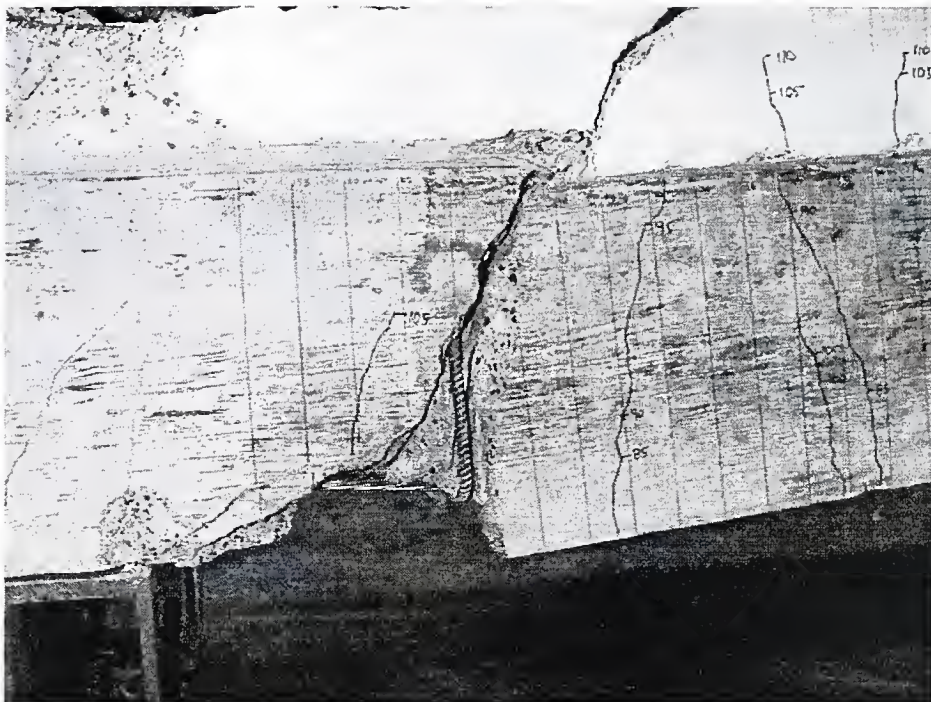
T-Beam FWC-6" Stirrup Spacing (South Face)
