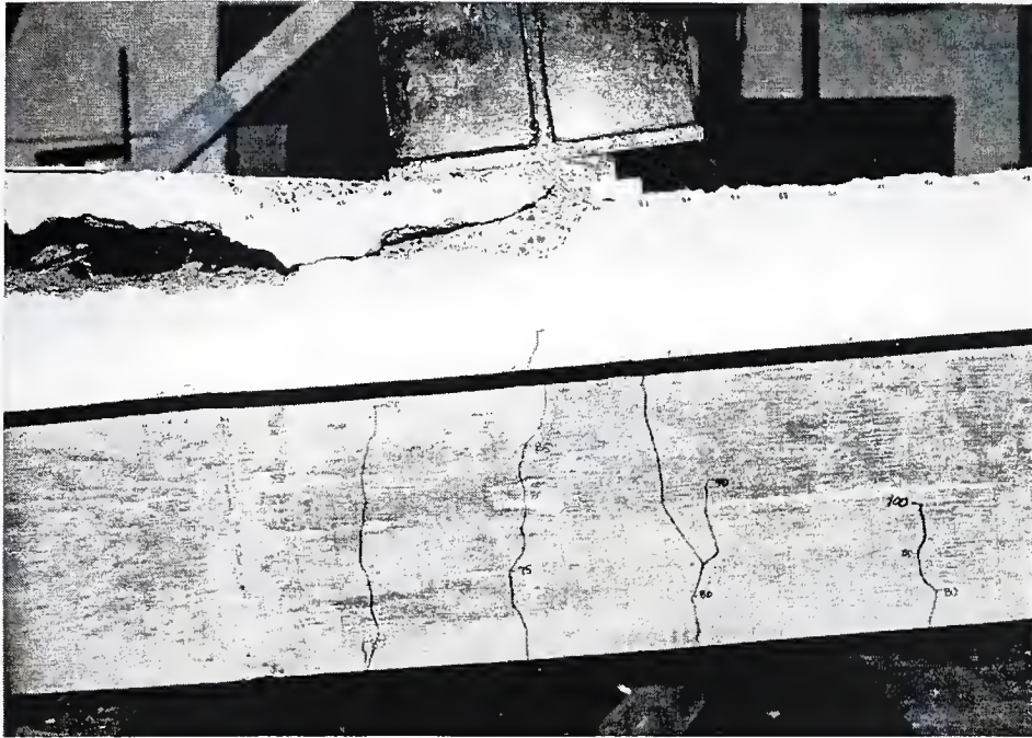
T-Beam FWC-15" Stirrup Spacing (South Face)
