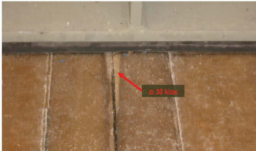
Figure 4.19: KSCI #P1b Test Specimen Damage at Longitudinal Joint Under Loading Beam
