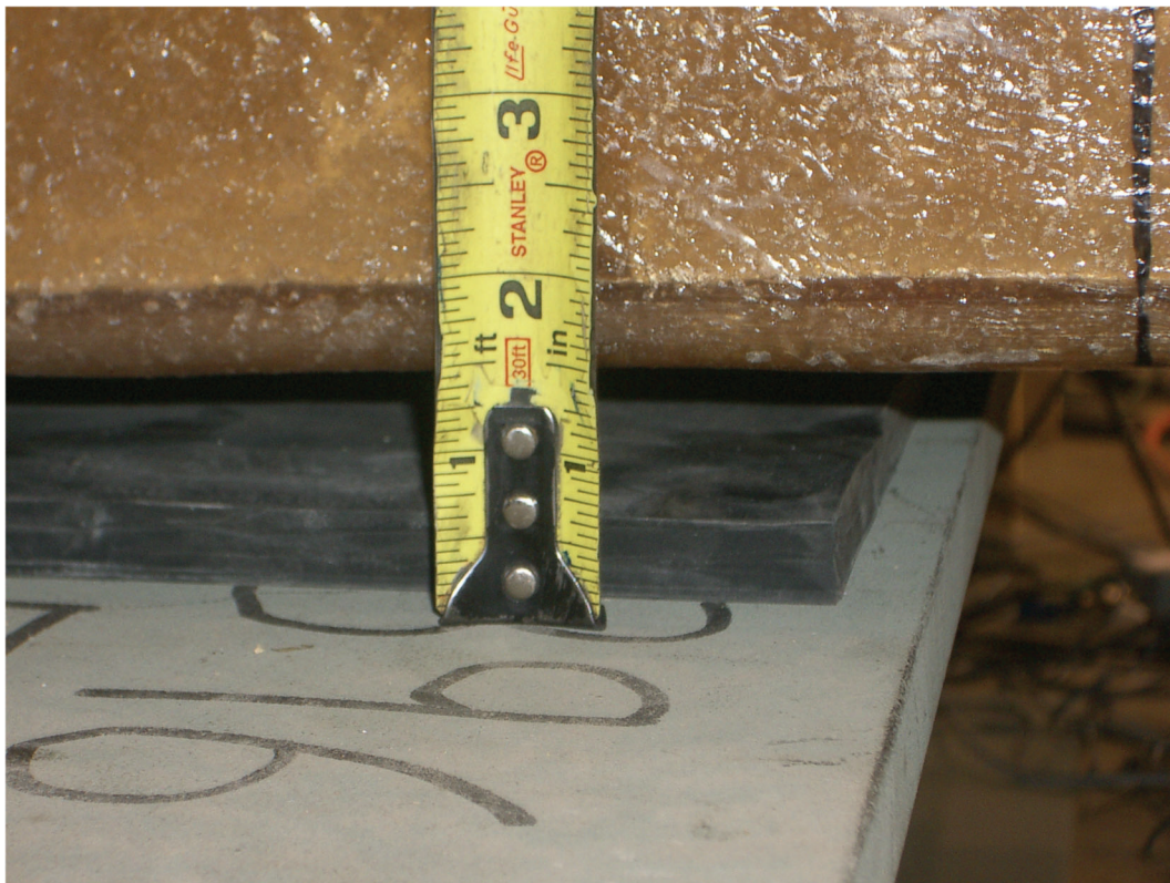
Figure 4.22: East side of the panel: 1 \frac{3}{8}'' (total gap) – \frac{1}{2}'' (neoprene thickness) = \frac{7}{8}''
