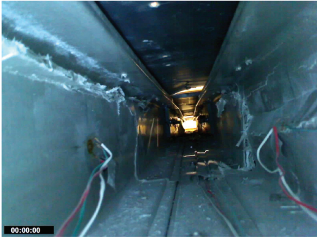
Figure 5.45: Damage to Deck Webs Under Load Patch
