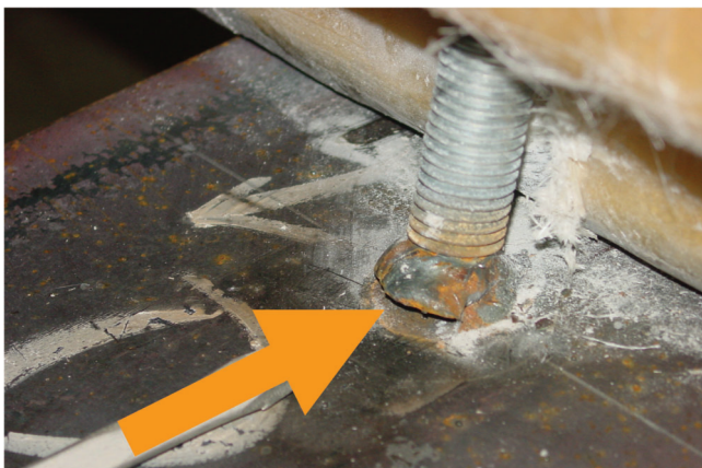
Figure 4.25: Detail of the Stud Connector After Test
