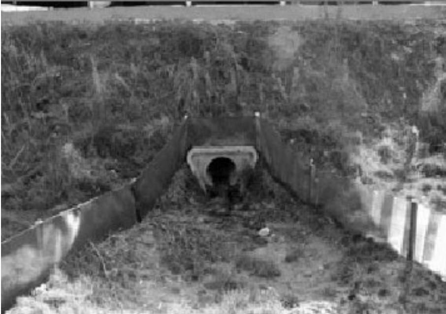
Figure 1. Small pipe culvert with mesh fence for small mammals and amphibians (Bank et al. 2002).
