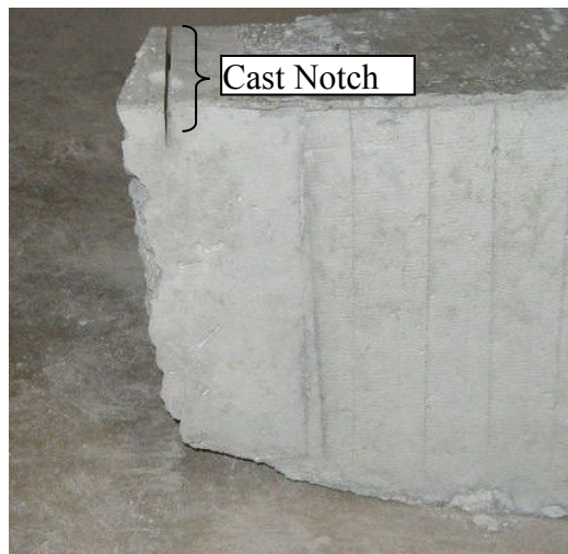
Figure 5.24: Crack propagation for specimen #24 which was cast with a 1.00" (D/8.5") notch and tested at 9 equivalent age hours
