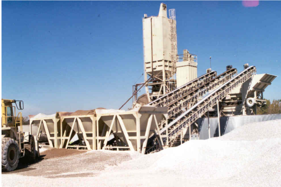
Figure 10-2 Batch Plant Aggregate Bins
