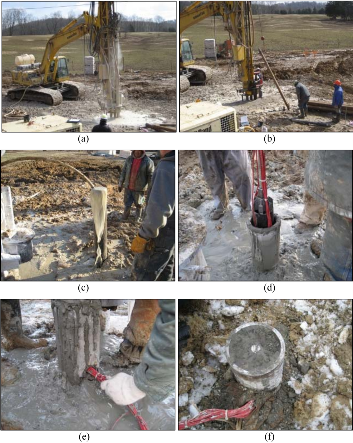
Figure 6.4 Installation of test pile: (a) drilling of the hole into the ground; (b) connecting the rod and casing; (c) grouting; (d) insertion of instrumented pipe; (e) positioning properly the instrumentation cables; (f) completed test pile
