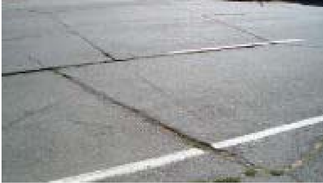
Figure 4: Reflective Cracking (after (8))
