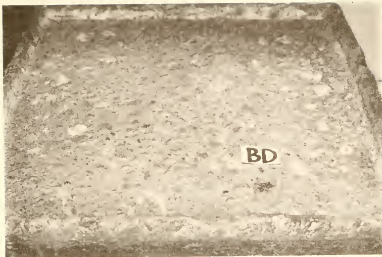
Figure 6.4.3 Appearance of Surface Condition of BD Concrete Pounded With 4% \text{CaCl}_2 Solution After Being Exposed Outdoors for 56 Weeks
