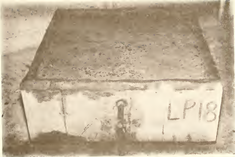
Figure 6.4.5 Appearance of Surface Condition of LPF Concrete Ponded with 4% \text{CaCl}_2 Solution After Being Exposed Outdoors for 56 Weeks
