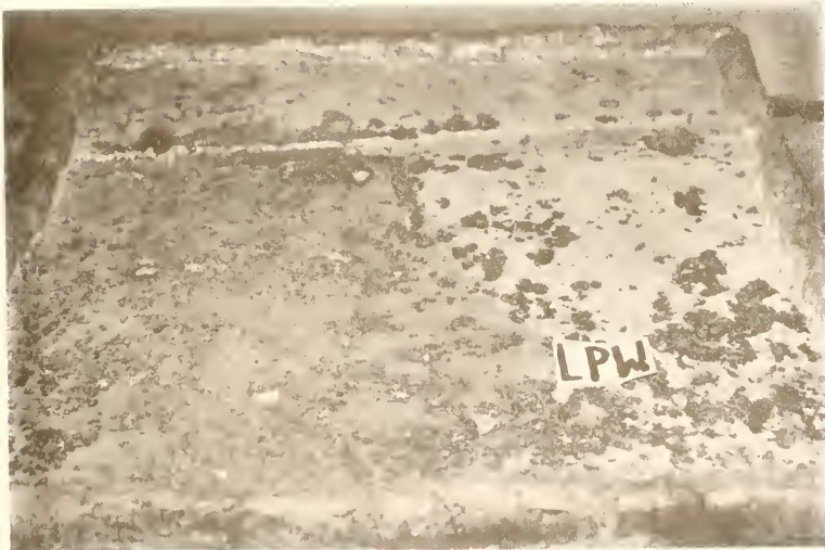
Figure 6.4.6 Appearance of Surface Condition of LPN Concrete Ponded With 4% \text{CaCl}_2 Solution After Being Exposed Outdoors for 56 Weeks
