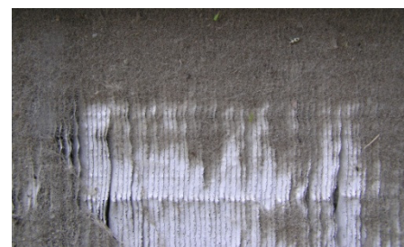
Figure 2 Field installed heat exchanger demonstrating large amount of fibrous loading
