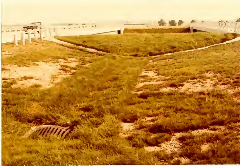
P.11 Slump areas where Wabash sod was used after 2-inch slitted drain pipe was placed to drain subgrade
