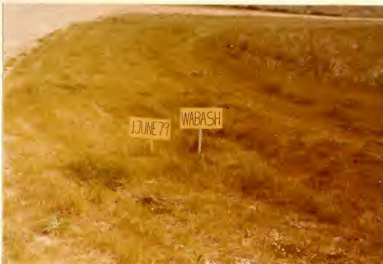
P.8 Wabash showing low turf cover where farm equipment has traffic over area. At very low nutrition.
