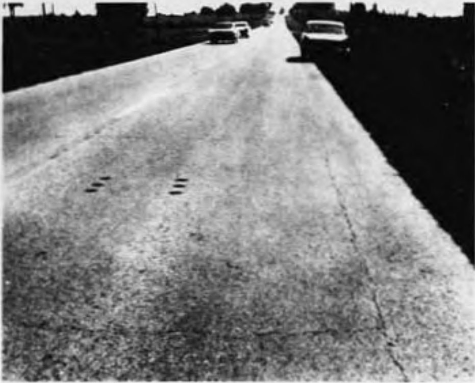
INDIANA 36 REFLECTION CRACKS
