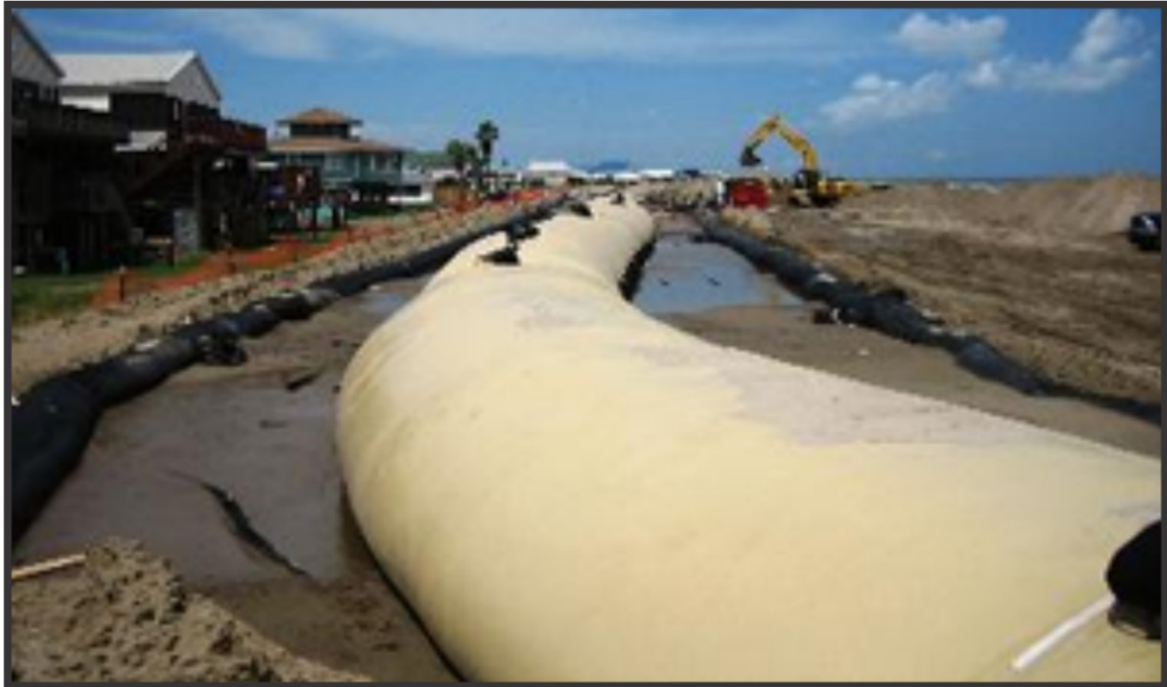
Figure 14. Example photo of a Geotube® used for sediment containment. Source: TenCate website.
