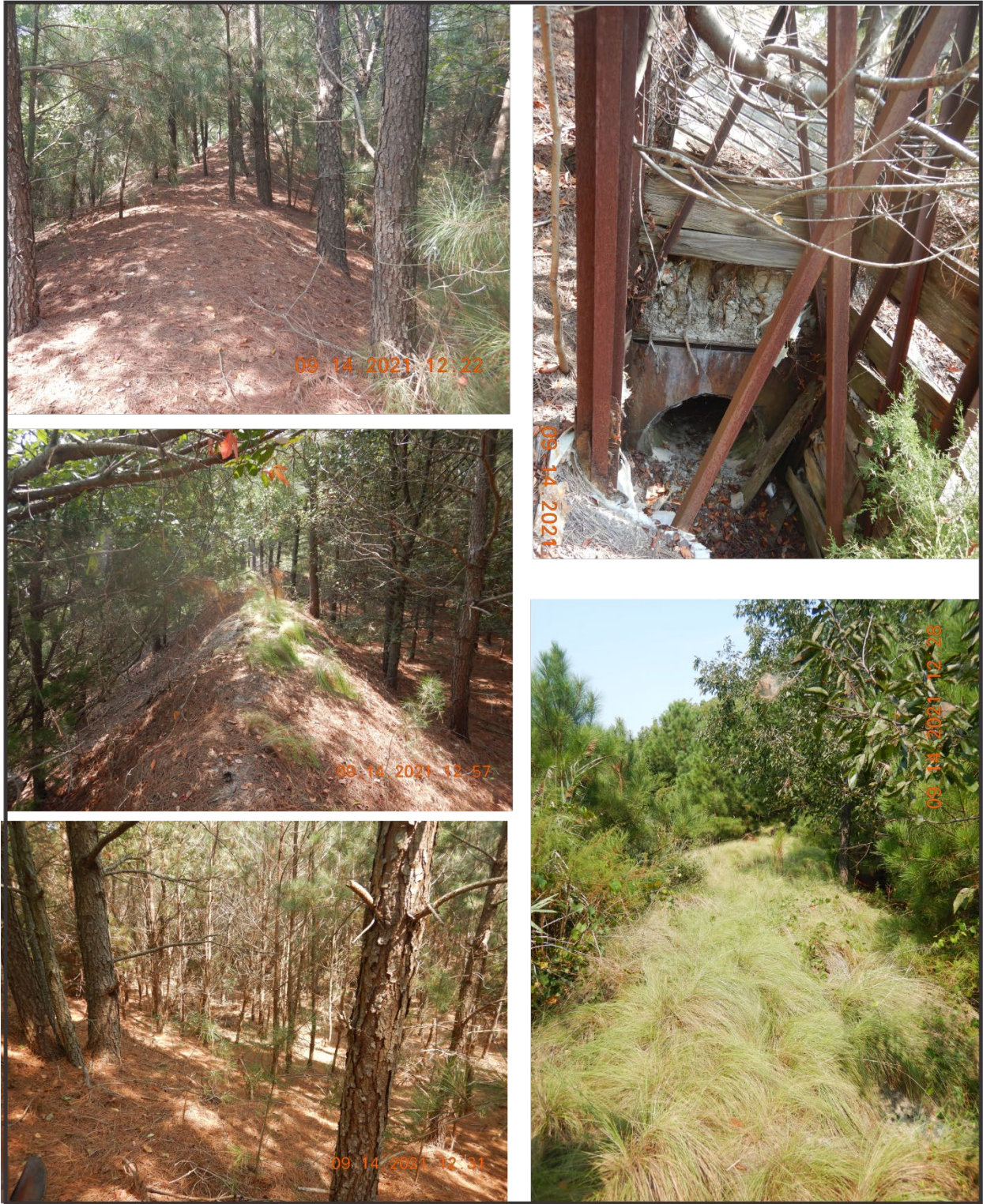
Figure 25. Ground photos showing the state of the berm and the outfall pipe. Photo credit: VIMS, Shoreline Studies Program.
