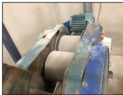
Figure 3-4. Roller crusher located at Gekko Pty Ltd
