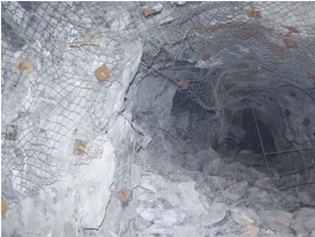
Figure 2.1 Stress-driven failure near the boundary of an excavation.
