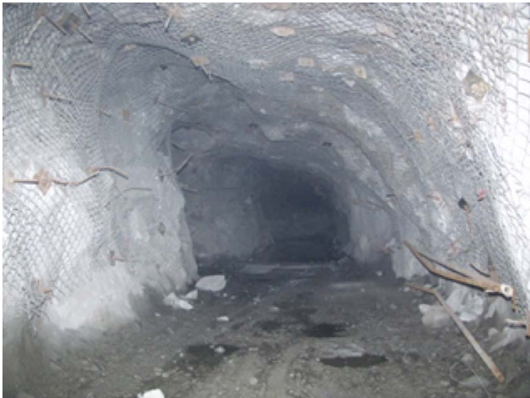
Figure 2.2 Notch created following stress-driven failure in a hard rock mine.
