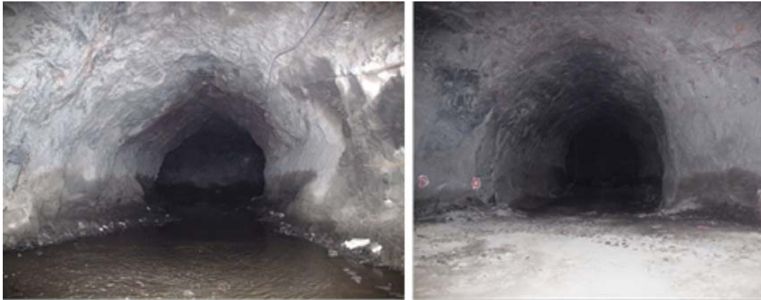
Figure 7.11 Full scale unsupported semi-circular tunnels showing on-set of brittle failure at the centre of the excavation roof due to high horizontal stress.
