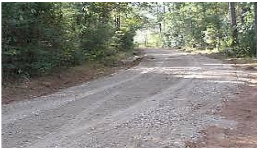
Figure 32: Road side gravel loss.
