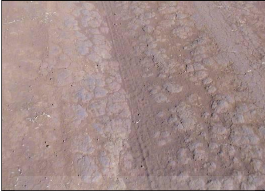
Figure 22: Road bed cracks.
