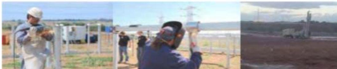
Figure 4.9.3: Photos of the mounting of frames for the PV panels in EIAR 23.
