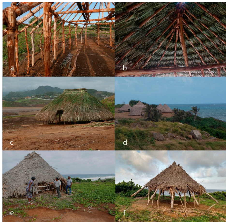
Figure 9. Experimental construction of a Kalinago roundhouse at Argyle, Saint Vincent in 2016, based on archaeological data from excavations at the site in 2009 and 2010; (a) configuration of an oval house (2016); (b) roof construction (2016); (c) finished oval house (2016); (d) overview of Argyle experimental village (2017); (e) decay of a round-house in 2019 (photos (a–e) by Menno Hoogland); (f) decay of a round-house in 2021 (photo by Augustine Sutherland).
