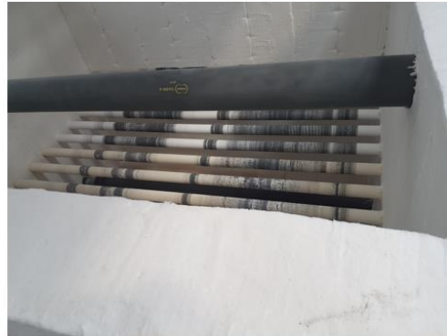
c) Contaminated rollers inside the furnace
