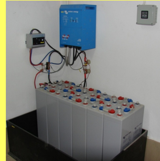
Fig. 4. View of accumulators' set, inverter and control charging device (photo D.Szyska)
