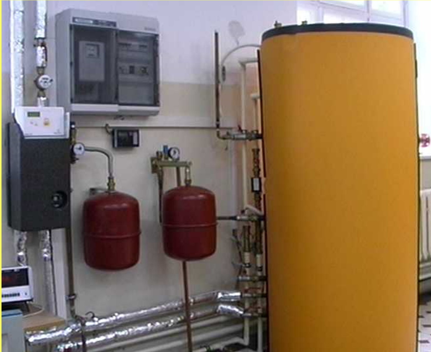
Storage tank, pump station and regulation of operating parameters in the system
