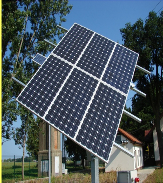
Fig. 2. View of mono-crystalline panel (photo D.Szyska)
