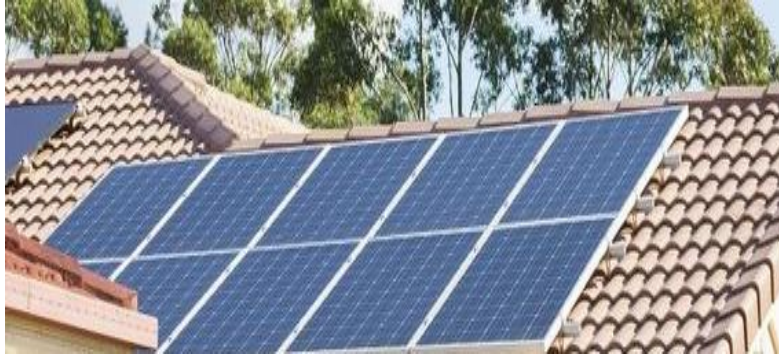
Figure 1. Roof-installed PV solar panels
