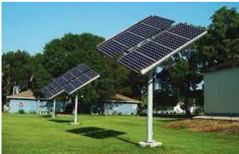
Figure 2. Pole installed solar modules [10]
