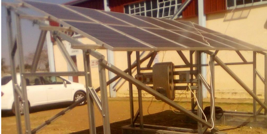
Figure 3. Ground- mounted solar PV modules at Capricorn TVET College
