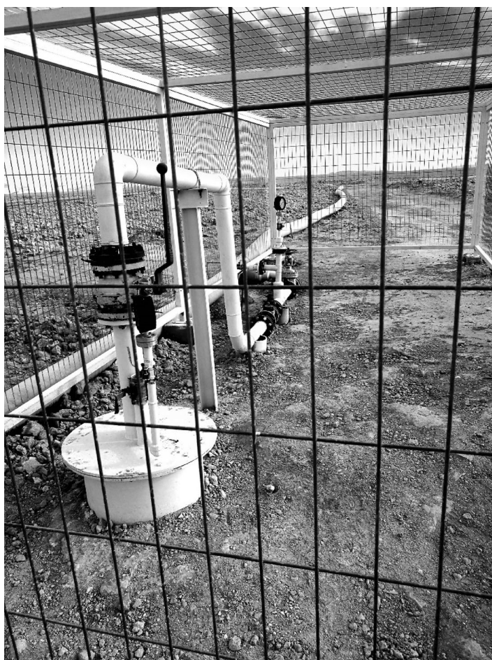
Figure 11. Mining pipelines in the Salar de Llamara (credit: Cristóbal Bonelli).
