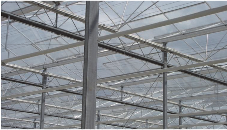
Figure 4. Glass greenhouse-galvanized steel frame (the Netherlands).
