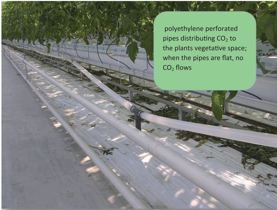
Figure 21. Plastic perforated pipes distributing CO 2 (The Netherlands).
