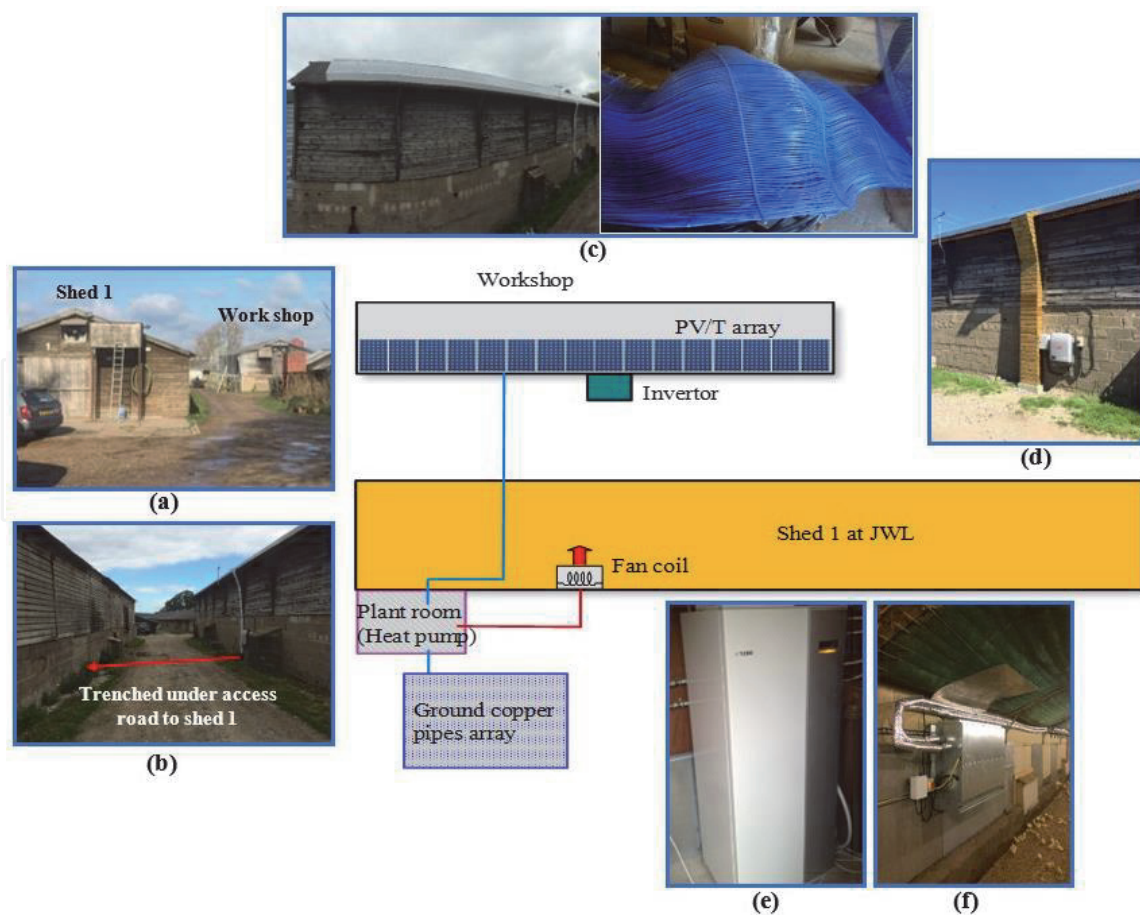
Figure 4. Hybrid renewable energy heating system installation: (a) workshop and shed 1; (b) trenched under access road to shed 1; (c) PV/T installed on the workshop roof; (d) inverter along with the external wall; (e) NIBE F1145 heat pump; (f) fan coil.
