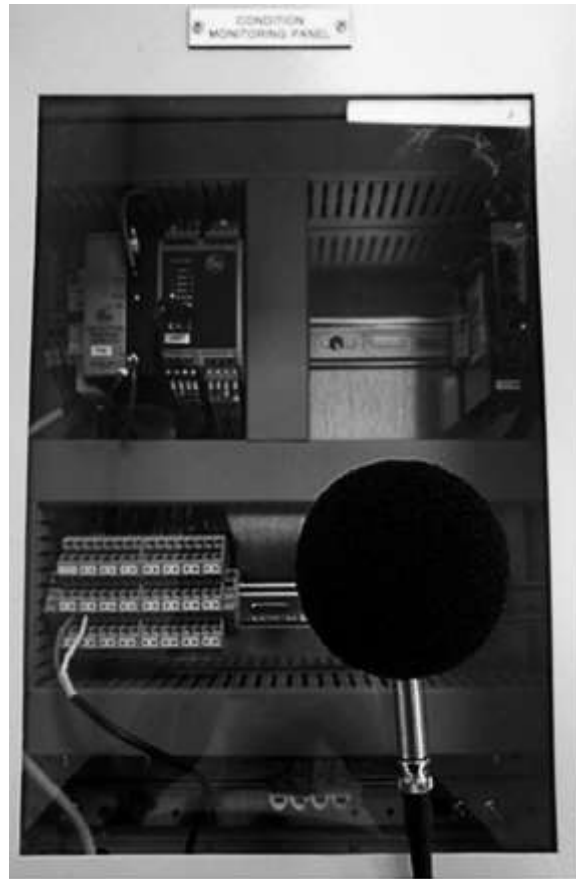
Figure 8. Signal acquisition unit and microphone used in this investigation by IFM electronics ltd.
