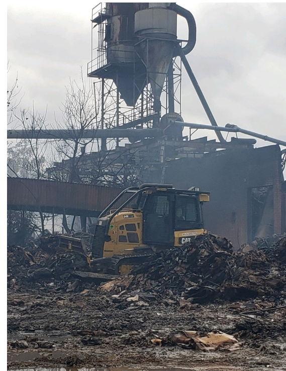
A Commission dozer pushes its way through the muck to spread debris out to be extinguished.
