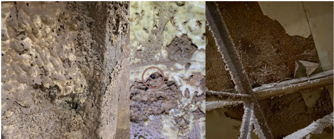
Fig. 4.10. Insulation damage to spray foam insulation and insulation panels inside a broiler house. Orange circle is highlighting an adult lesser mealworm, Alphitobius diaperinus , inside the damaged insulation. Images taken by B. Lyons
