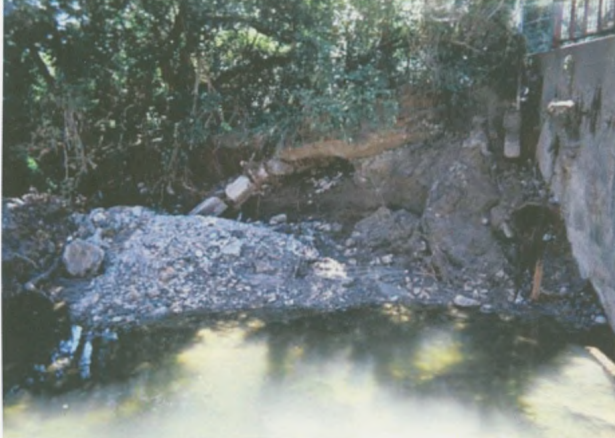
August 26, 2005: Storm Damage
