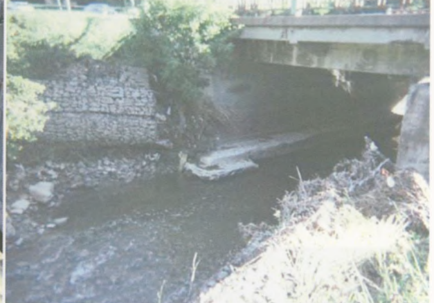
September 1, 2005: View of Crossing, Storm Impact
