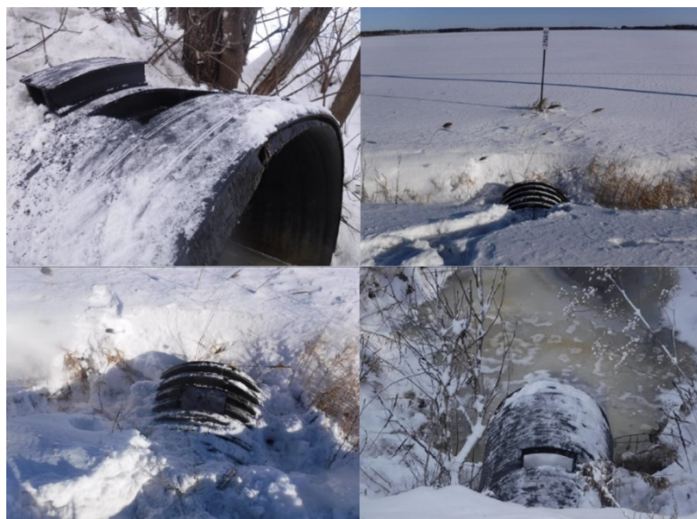
Figure 6.1 HDPE pipes in field service in Quebec
